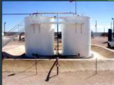
▶ Lined Containment Dike
