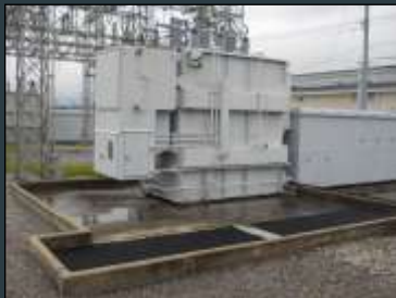
▶ Concrete Curbing Draining to a Concrete Basin
